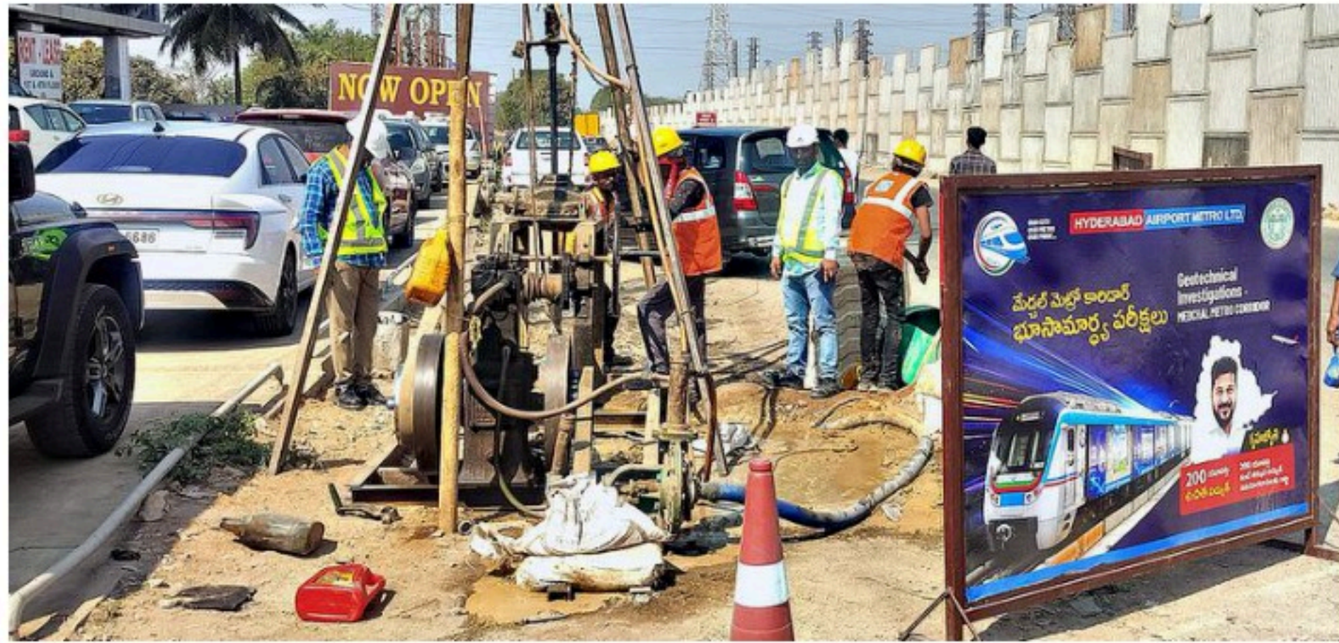
Hyderabad Airport Metro Limited begins underground testing for the proposed metro rail connectivity towards Medchal and Shamirpet on Sunday
