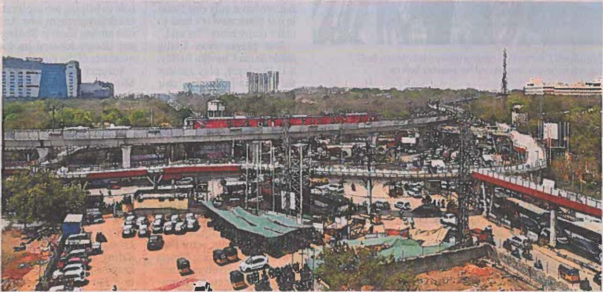
Works on the skywalk at the busy Uppal junction are on at a brisk pace. — Photo: Surya Sridhar
