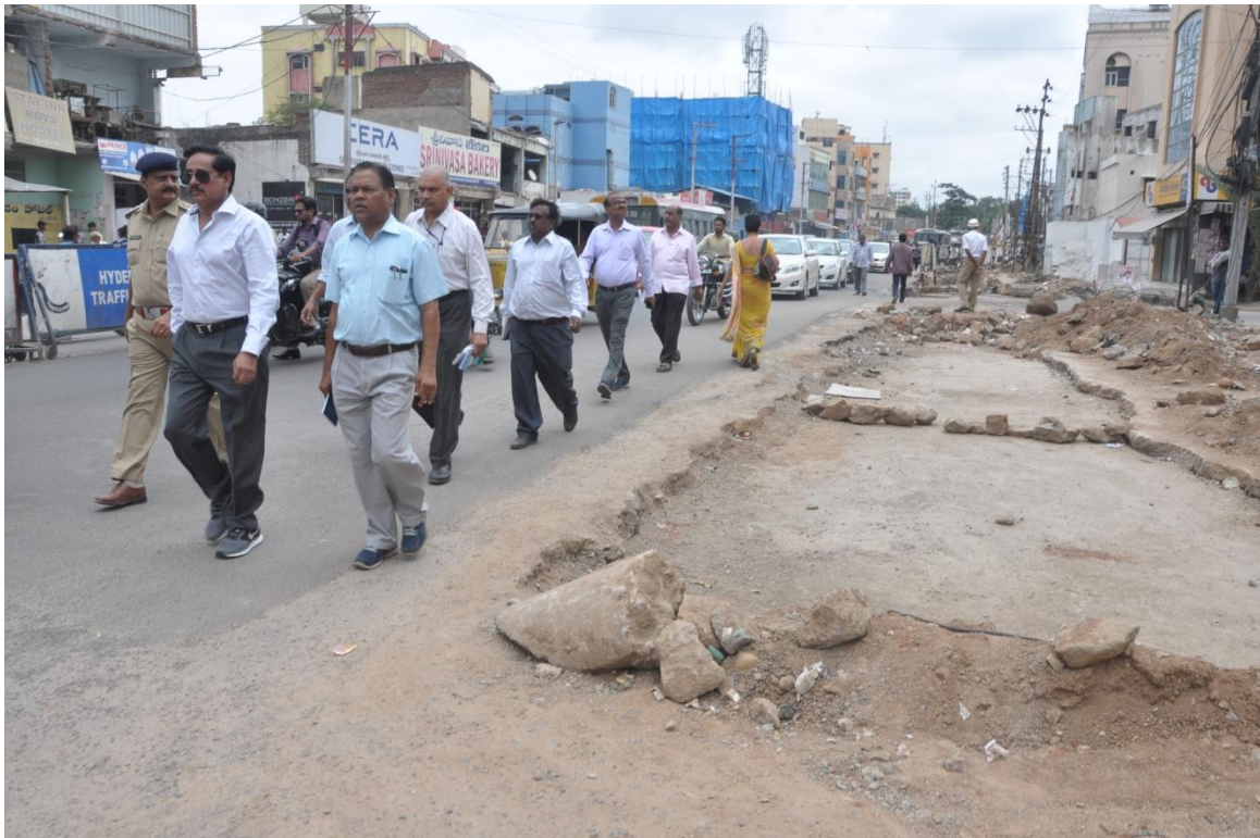
MD, HMR Mr. NVS Reddy inspecting the road restoration works of Metro corridor-II in Musheerabad on Thursday (July 30, 2015)
