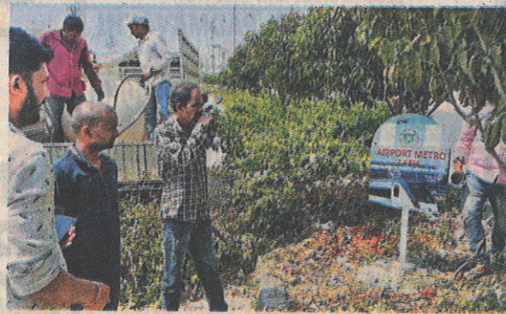
Workers install markers along the proposed route for Hyderabad Airport metro, at Nanakramguda road on Tuesday.
