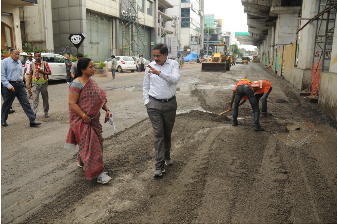
MD, HMRL Mr. NVS Reddy inspecting road restoration works on Road No. 36 in Jubilee Hills on Friday (23.09.2016).
