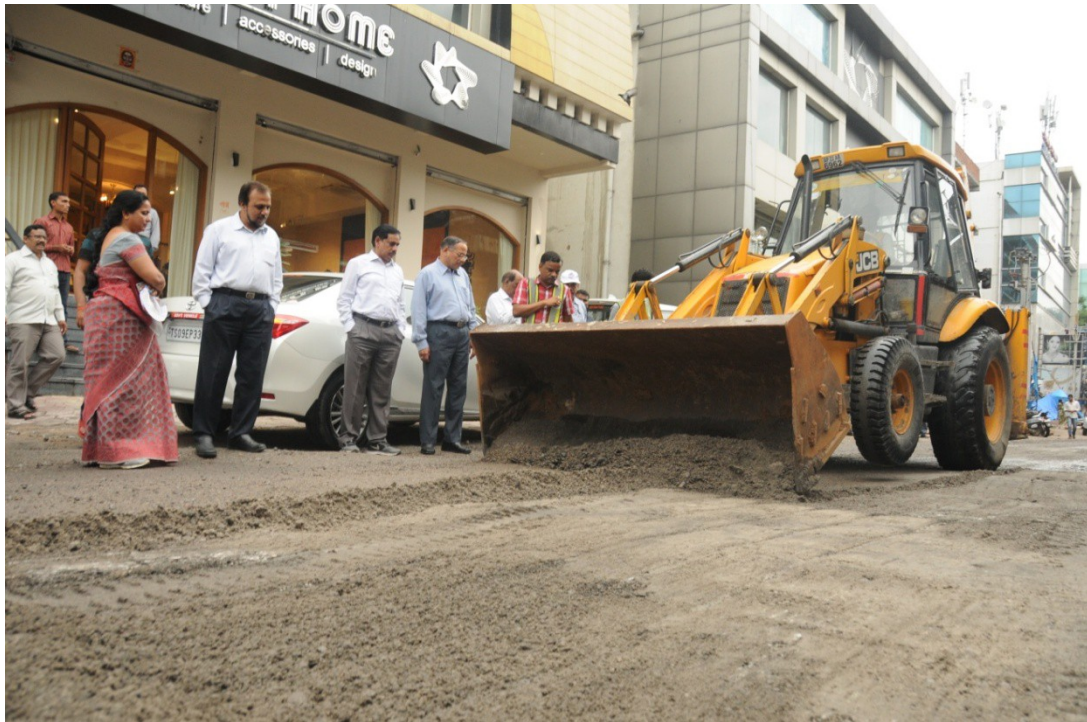
MD, HMRL Mr. NVS Reddy inspecting road restoration works on Road No. 36 in Jubilee Hills on Friday (23.09.2016)
