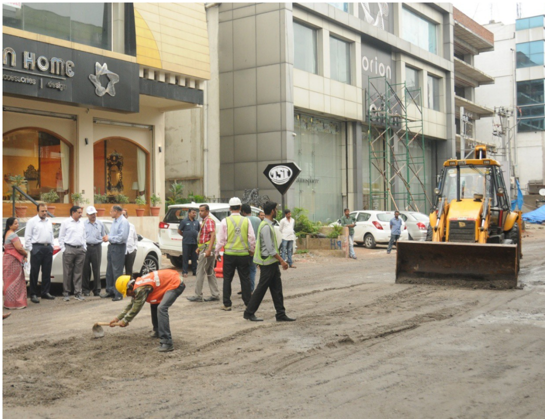
MD, HMRL Mr. NVS Reddy inspecting road restoration works on Road No. 36 in Jubilee Hills on Friday (23.09.2016).
