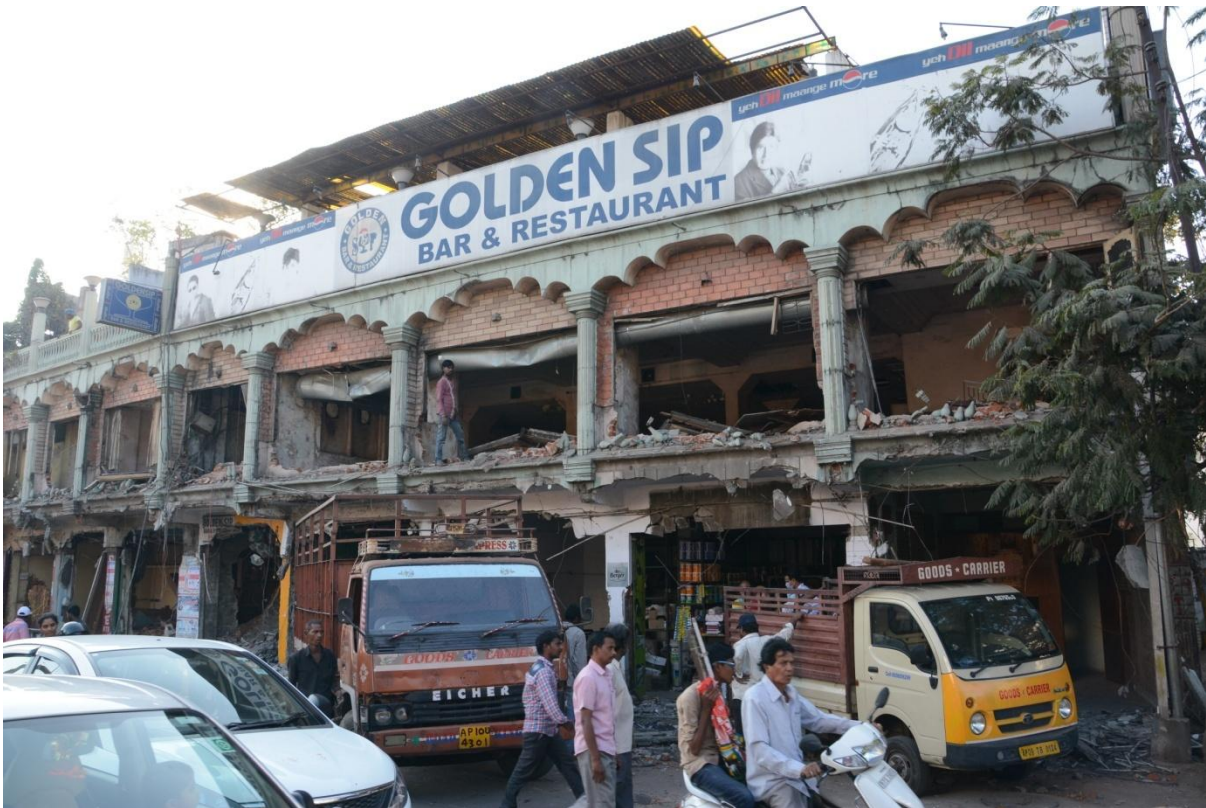
Dismantling of Golden Sip Hotel in progress at Musheerabad junction on Metro Rail Corridor II on Saturday (January 21, 2017)
