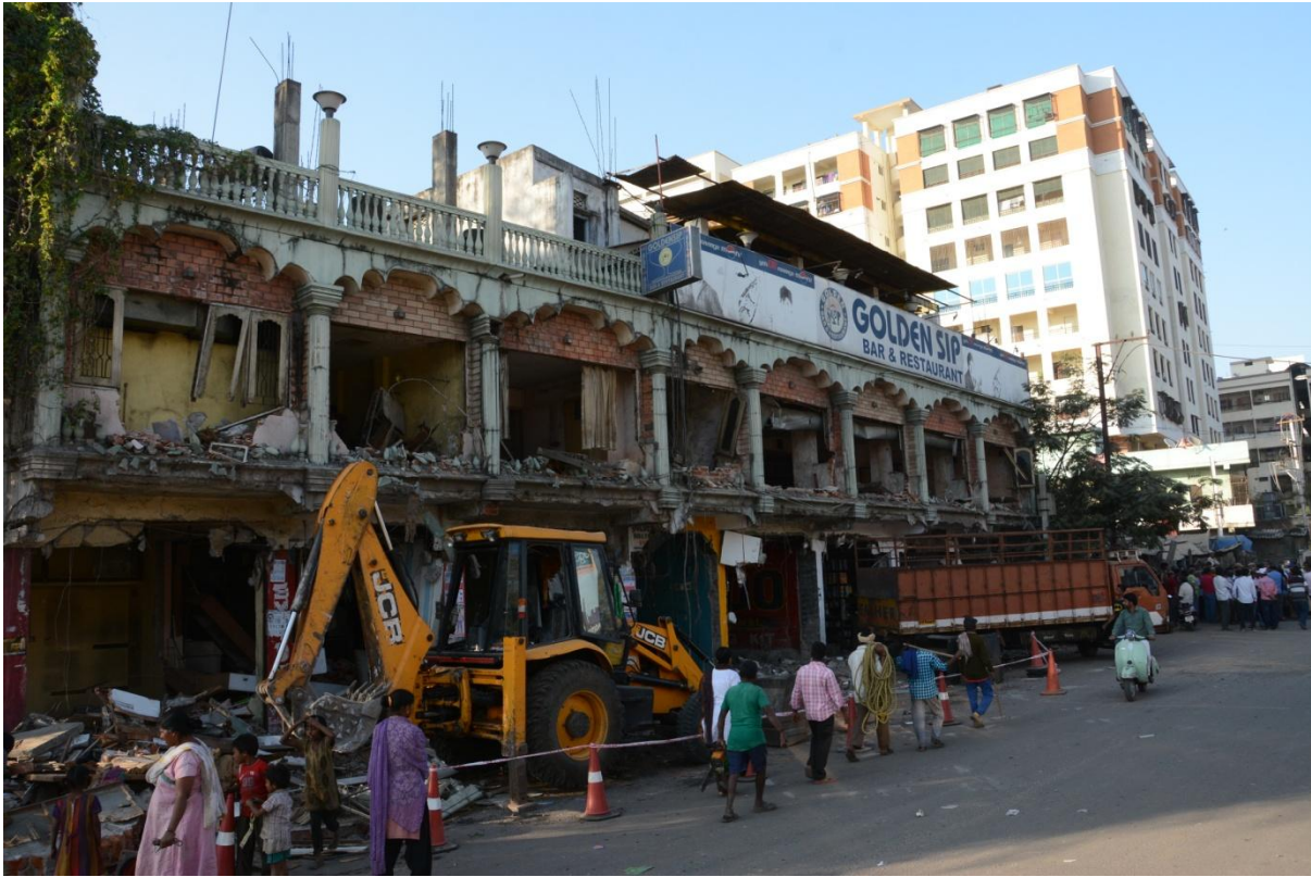
Dismantling of Golden Sip Hotel in progress at Musheerabad junction on Metro Rail Corridor II on Saturday (January 21, 2017)
