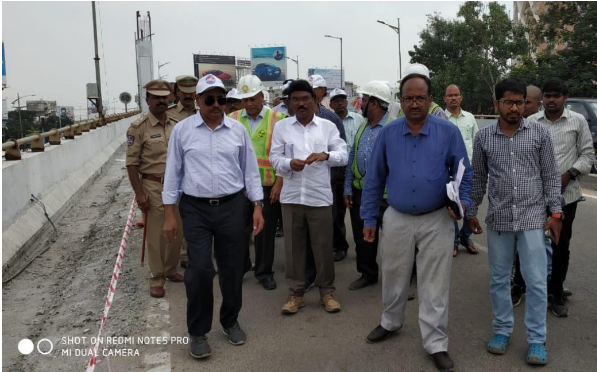
MD, HMRL Mr.NVS Reddy along with Metro Rail engineers inspecting the widening work of Hitec City Flyover (ramp portion) on Sunday (30.09.2018)
