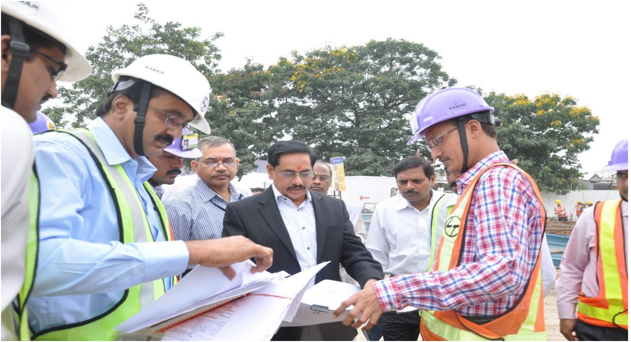
MD, HMR Mr. NVS Reddy inspecting the construction works at Metro Rail interchange station at Imlibun along with engineers of HMR and L&TMRHL at MGBS on Monday (November 16, 2015)
