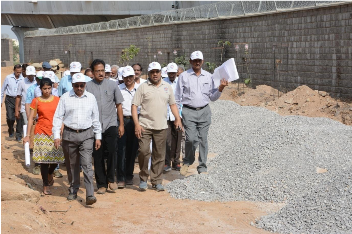
MD, HMRL Mr. NVS Reddy inspecting the ongoing streetscaping works near Miyapur Metro Rail station on 29.04.2017 (Saturday)
