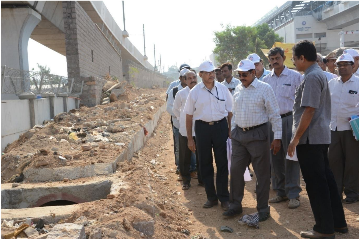
MD, HMRL Mr. NVS Reddy reviewing the progress of stormwater drainage works near Miyapur Metro Rail station on 29.04.2017 (Saturday)
