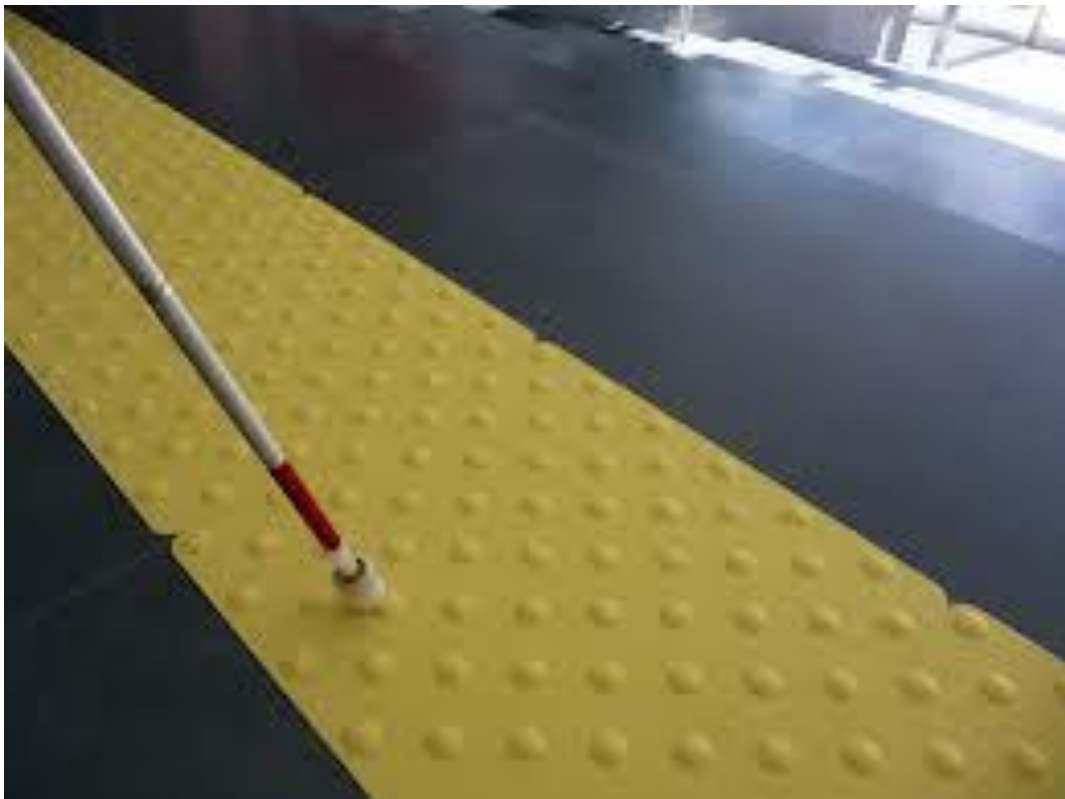
Figure 4: Tactile strip at Metro stations to guide blind people
