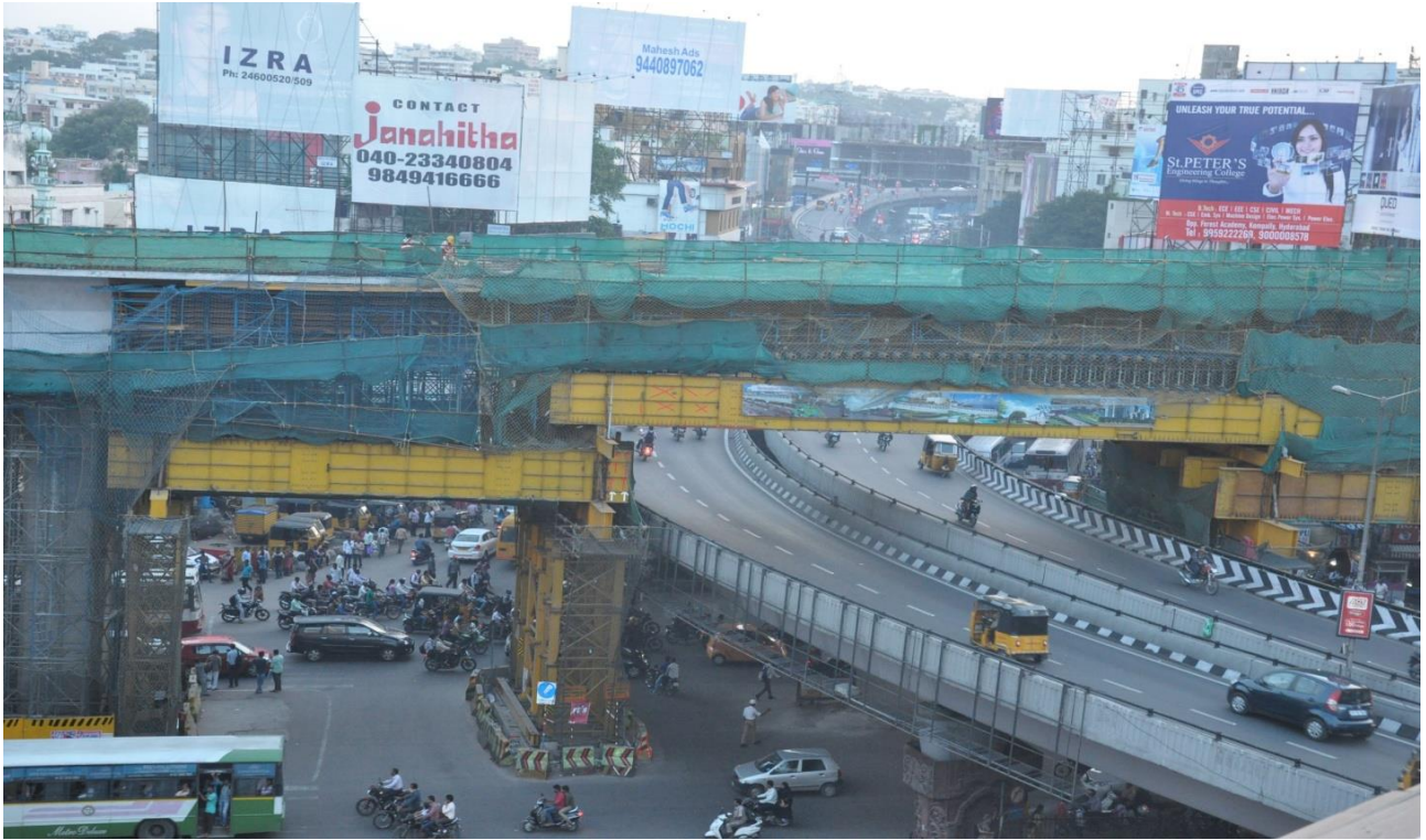
Arrangements made for traffic movement from Begumpet to Banjara Hills and on flyover (during construction)
