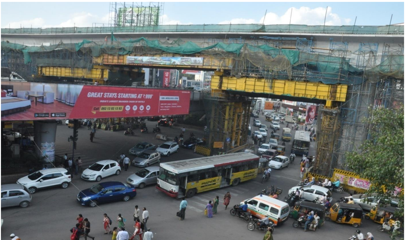
Arrangements made for traffic movement from Banjara Hills to Begumpet (during construction)
