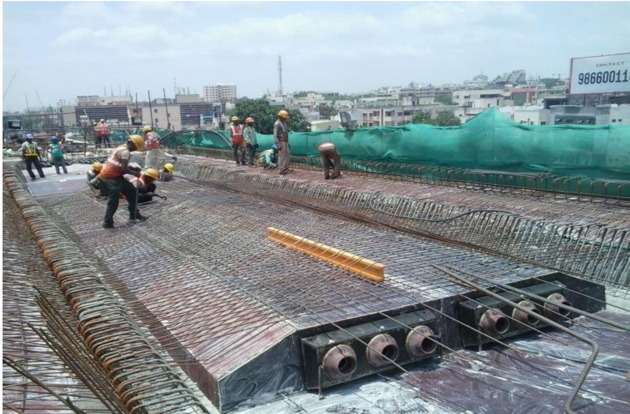
Reinforcement for top slab is in progress for cast In-situ span (during construction)
