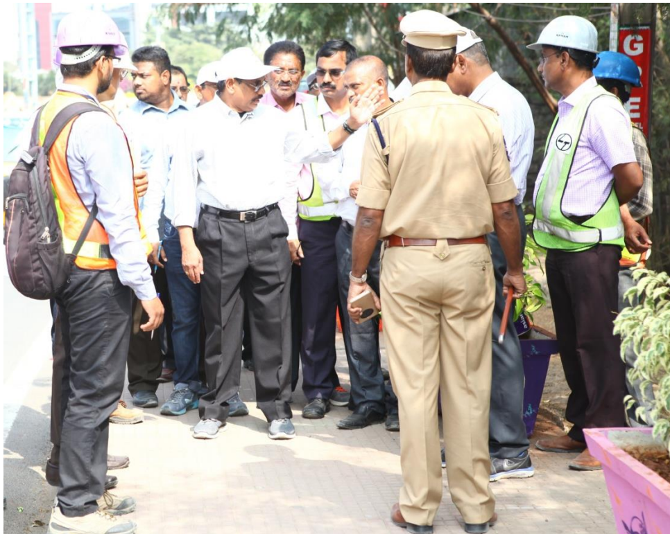
MD, HMRL Mr.NVS Reddy instructing HMRL and L&T engineers to locate foundations adjacent to Cyber Towers on Thursday (December 07, 2017)
