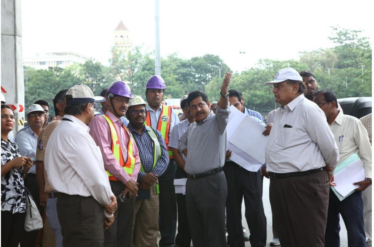
HMRL MD Mr.NVS Reddy instructing LTMRL engineers for construction of skywalk for entry exit towards Telangana State Archaeology Museum side on 04.07.2018 (Wednesday)
