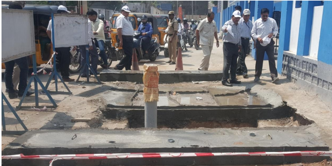
HMRL MD Mr NVS Reddy inspecting the RWHS near Institute of Engineers, Khairatabad
