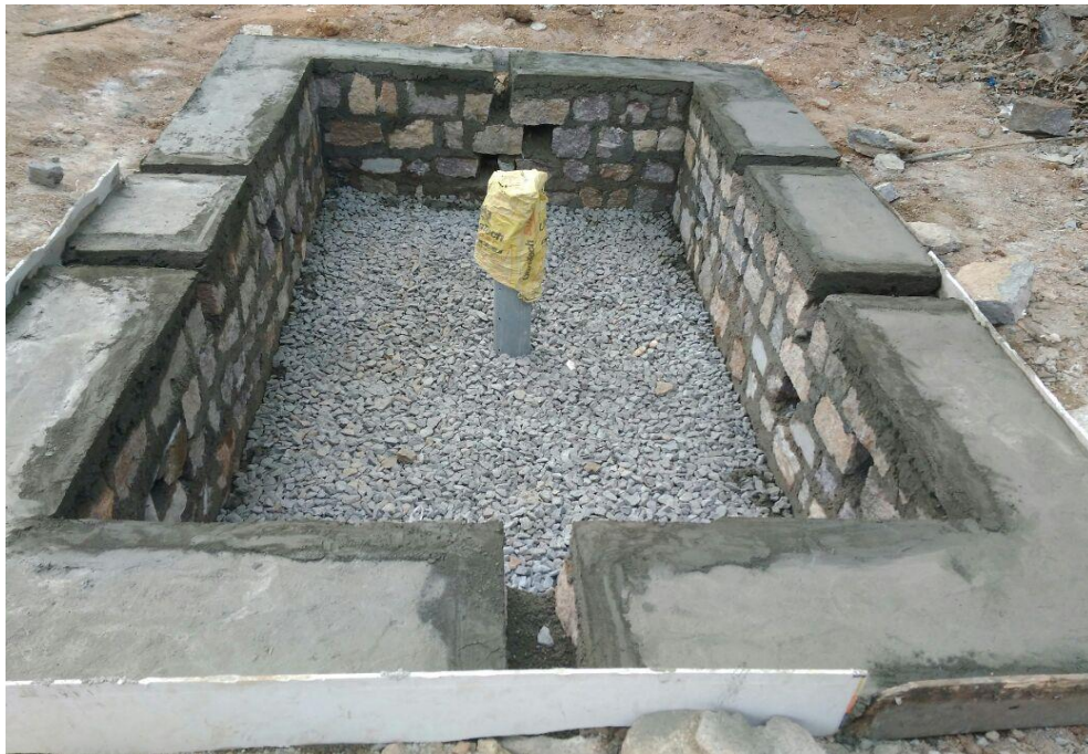
Filling of 40 mm HBG metal in RWHS near Institute of Engineers, Khairatabad
