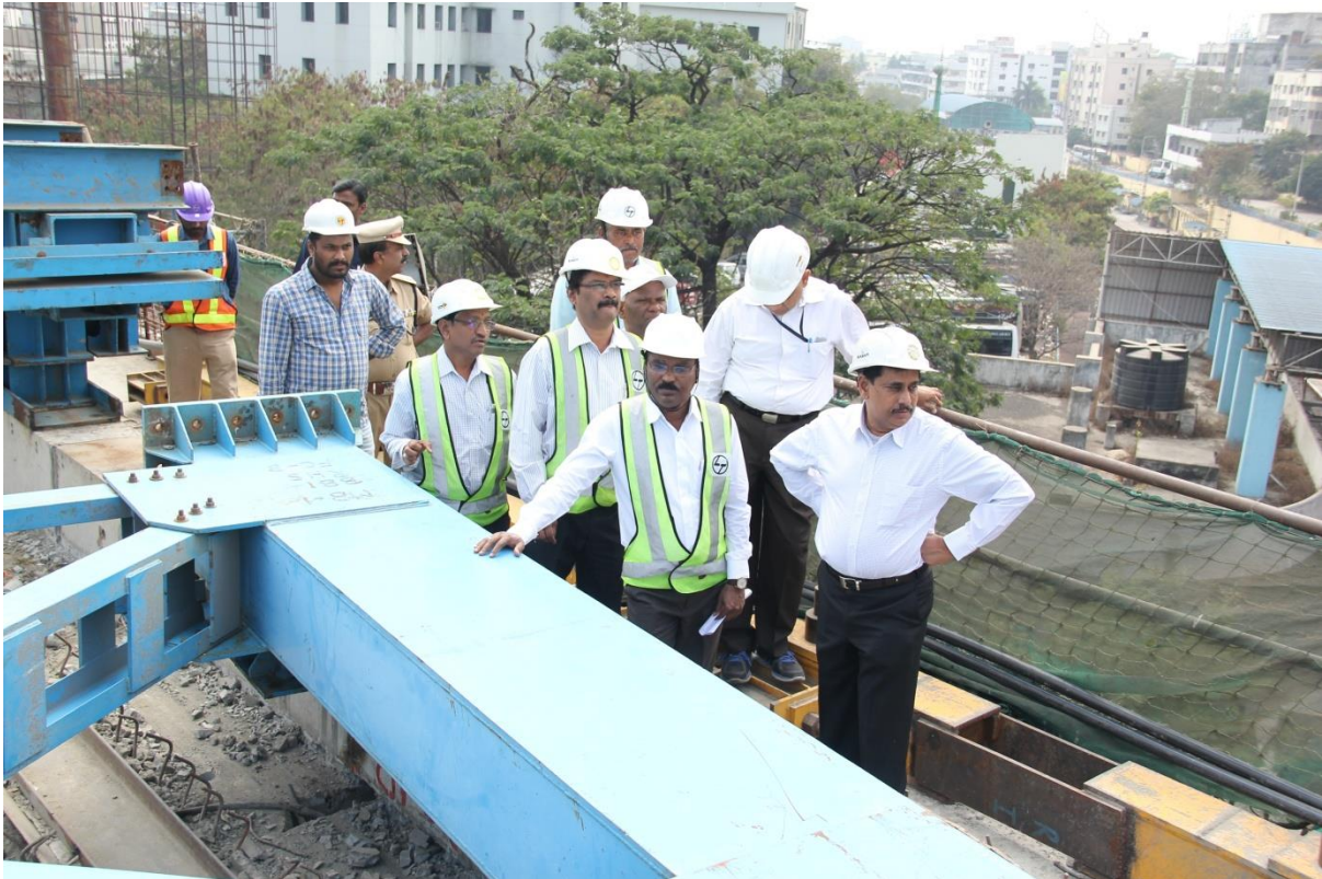
MD, HMRL Mr.NVS Reddy inspecting the 'Bridge Builder' used for constructing the Metro ROB at Lakdi-ka-pul on Sunday (February 11, 2018)
