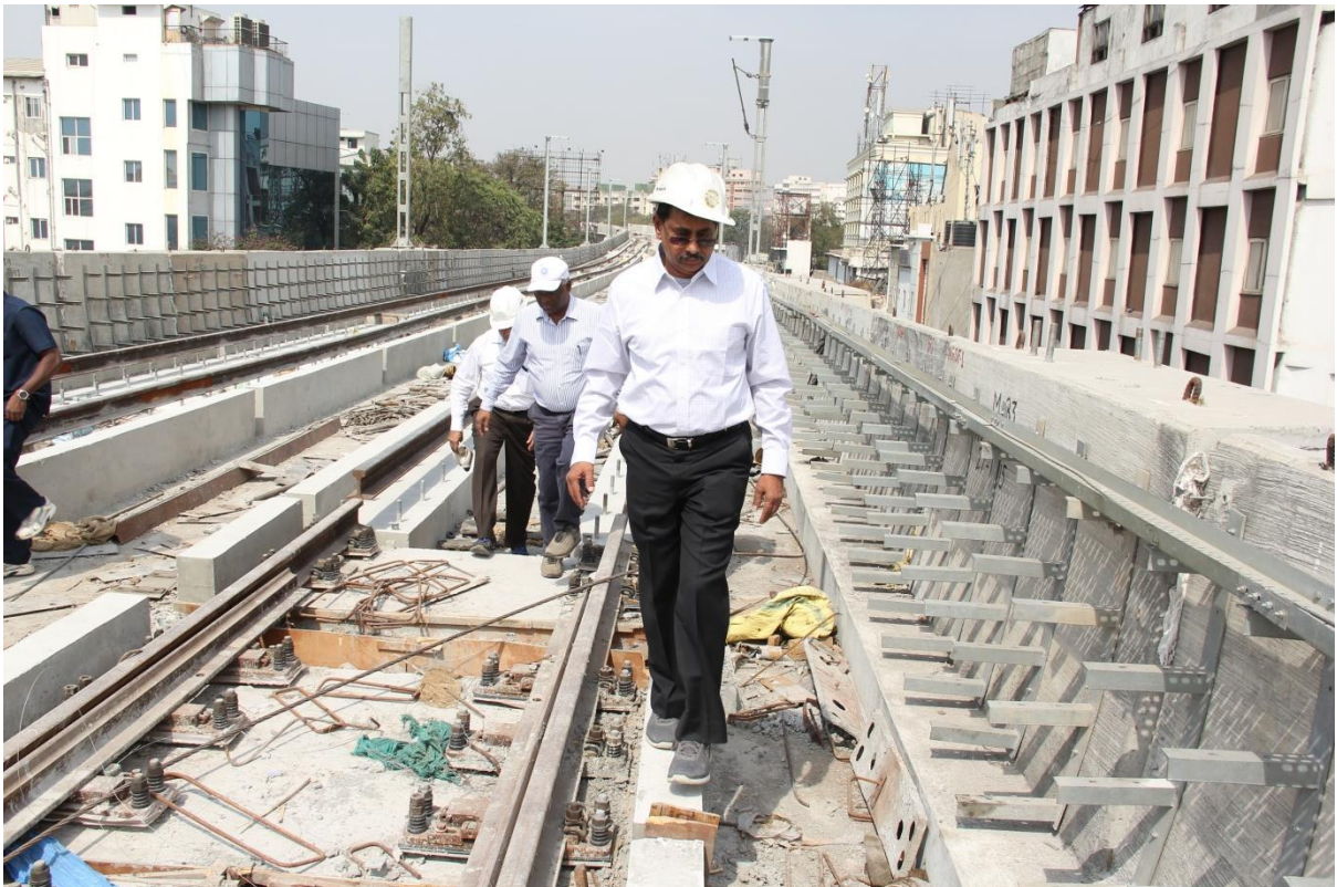
MD, HMRL Mr.NVS Reddy inspecting the track works on the viaduct connecting ROB at Lakdi-ka-pul on Sunday (February 11, 2018)
