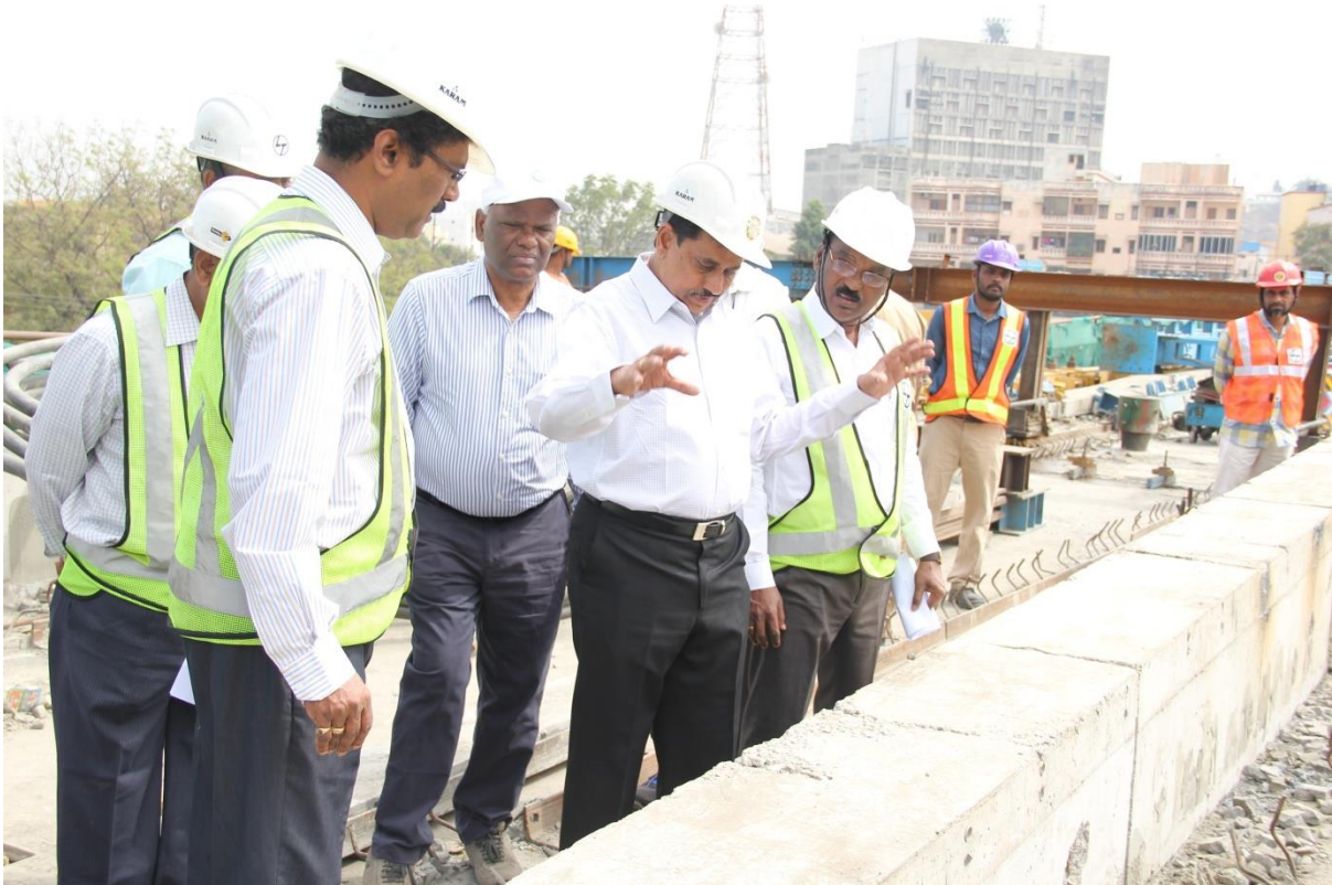
MD, HMRL Mr.NVS Reddy interacting with L&T bridge engineers on top of the Lakdi-ka-pul ROB on Sunday (February 11, 2018)
