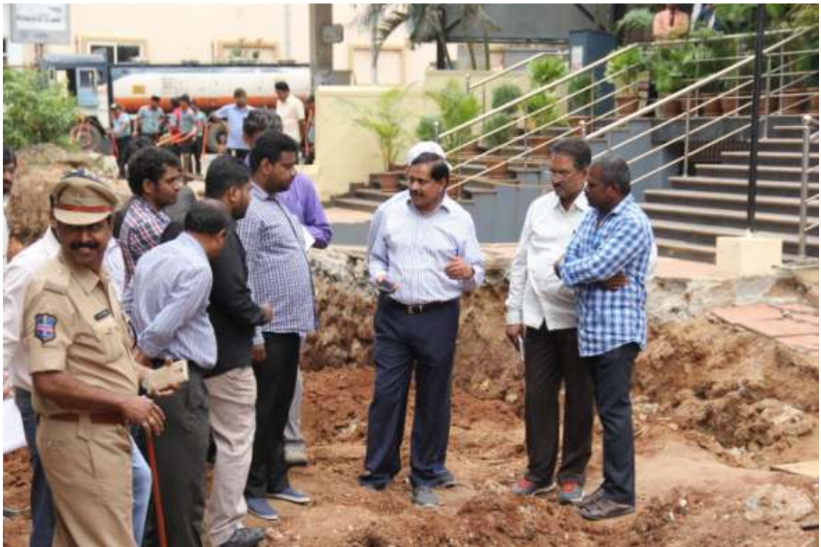
MD, HMRL Mr. NVS Reddy inspecting service road formation and other urban rejuvenation works at JNTU Metro station on Monday (02.10.2017)
