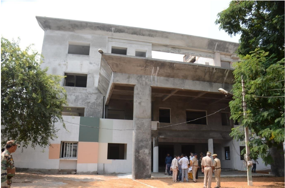
A view of Sainik Aram Ghar being constructed by HMRL at old Gandhi hospital premises
