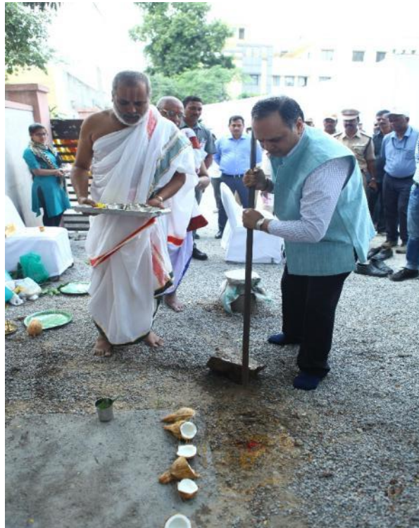
Chief Secretary Dr.S K Joshi performing Bhoomi Pooja (Ground Breaking Ceremony) for the Multilevel parking project at Nampally today (08-09-2018)
