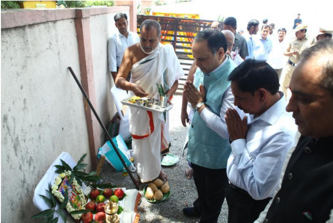
Chief Secretary Dr.S K Joshi and MD, HMRL Mr.NVS Reddy Performing Bhoomi Pooja (Ground Breaking Ceremony) for the Multilevel parking project at Nampally today (08-09-2018)
