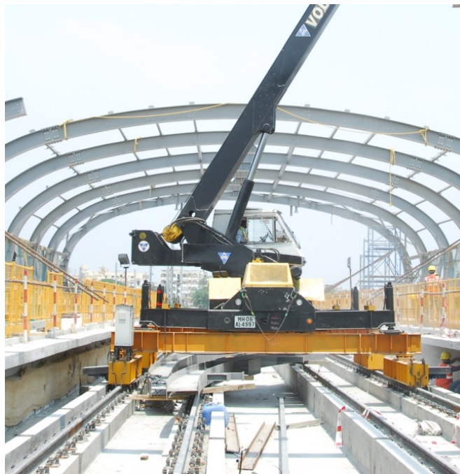
Crane used for erecting Metro station roof trusses (innovative construction method to avoid crane operation from road level).
