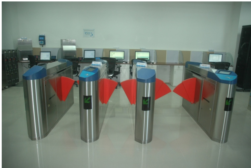
Automatic Fare Collection (AFC) gates - "State-of-the-Art" Ticketing system and Passenger control
