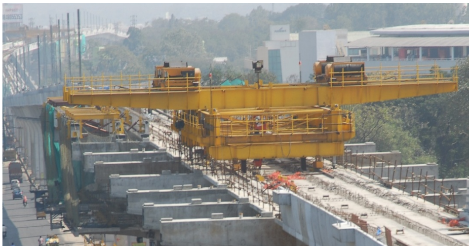
Gantry used for erecting wings of Metro station (innovative construction method to allow free flow of traffic on the road below).
