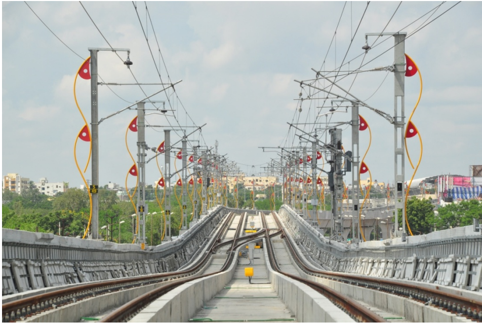
Hyderabad Metro Rail Over Head Electrification (OHE) Masts on elevated viaduct.
