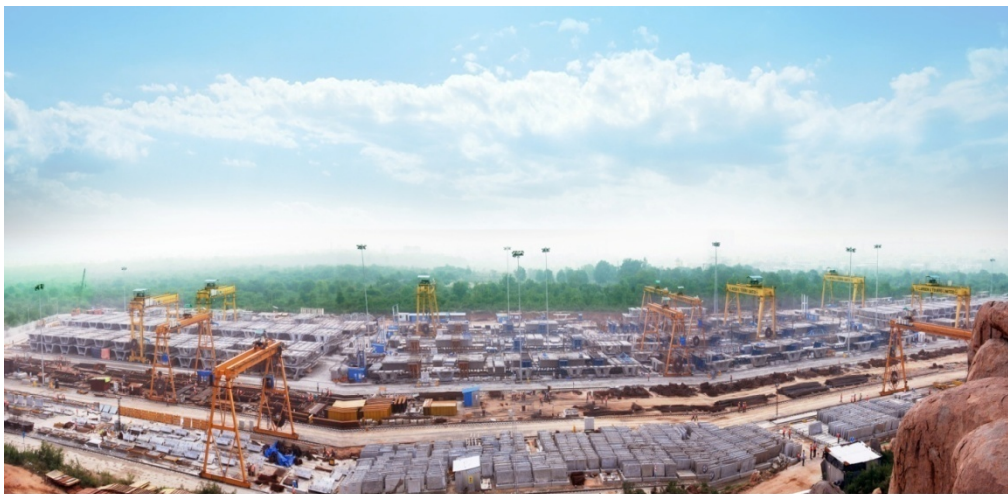
The panoramic view of Qutubullapur precast yard (64 acres- India's second biggest urban precast yard).
