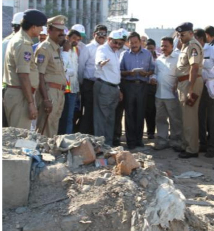
MD, HMR Mr. NVS Reddy instructing engineers to immediately take up road restoration works at MJ market on Saturday (February 07, 2015)
