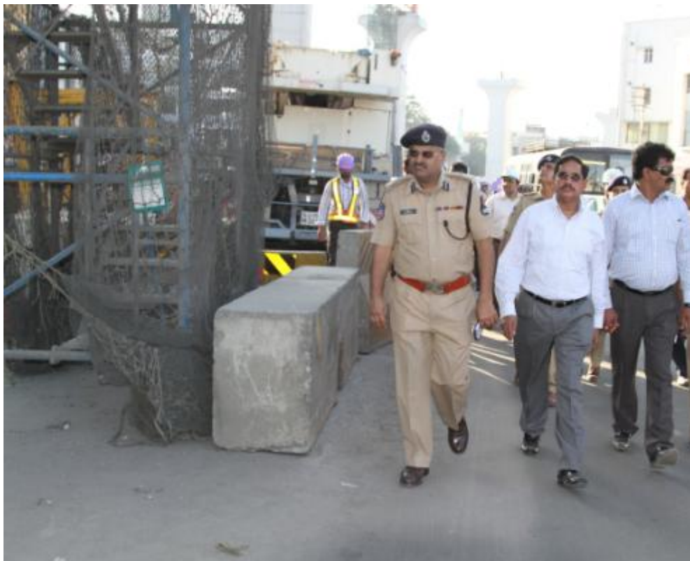
MD, HMR Mr. NVS Reddy conducting inspection with Additional CP (Traffic), Hyderabad Mr. Jitender on road restoration works at Malakpet on Saturday (February 07, 2015)
