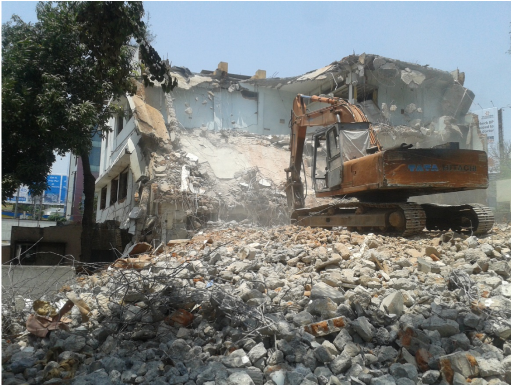
Nandini cafe/Goutham Reddy property at Jubilee Hills check post being demolished by HMR to facilitate Metro viaduct construction in sharp curve
