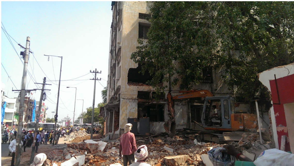
Multi-storied railway property near Secunderabad station being demolished by HMR for construction of Secunderabad East Metro station
