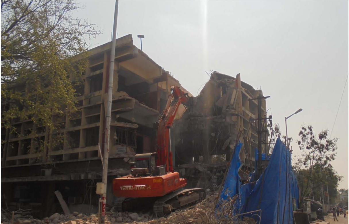
Dismantling a part of BHEL building at Secunderabad clock tower in corridor-II
