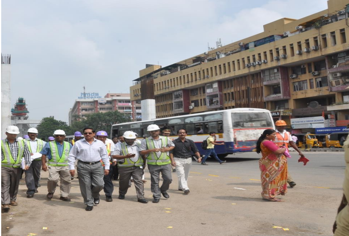
MD, HMR Mr. NVS Reddy inspecting ongoing Metro Rail Interchange terminal works at Ameerpet junction
