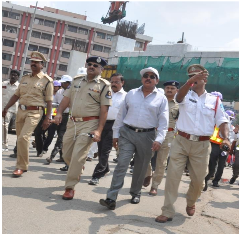
MD, HMR Mr. NVS Reddy along with Addl CP (Traffic), Mr. Jitender, inspecting ongoing Metro Rail works and traffic movement in Yousufguda
