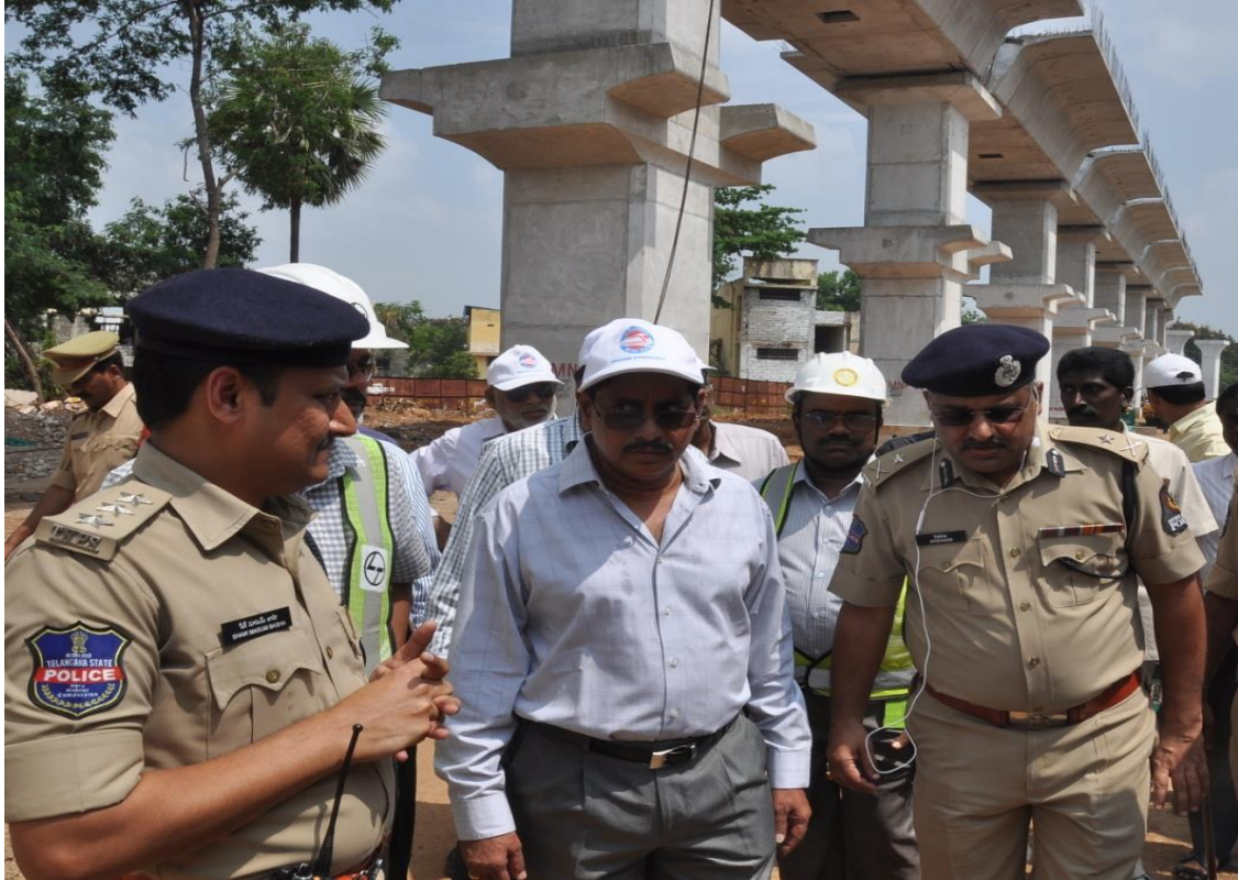
MD, HMR Mr. NVS Reddy along with Addl CP (Traffic), Mr. Jitender, inspecting ongoing Metro Rail works and traffic movement in Yousufguda
