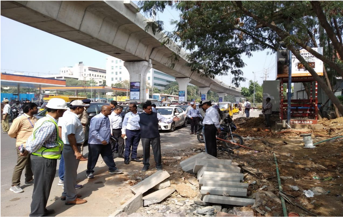
MD HMRL, NVS Reddy inspecting Raidurg station on Friday (22-11-2019) along with HMRL and L&THMRL engineers.
