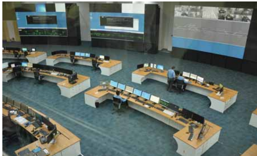
Inside view of Command Control Centre
