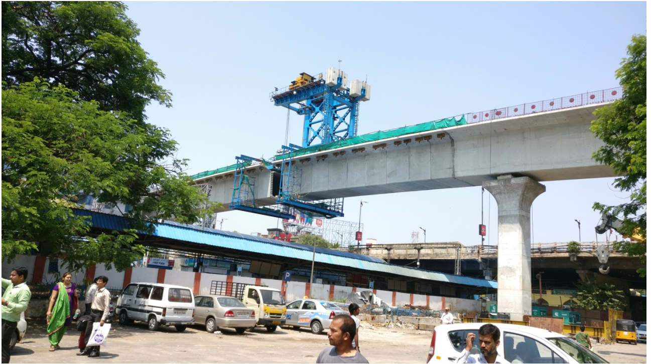
Begumpet Metro ROB construction over the Railway station using specially designed 'Bridge Builder'
