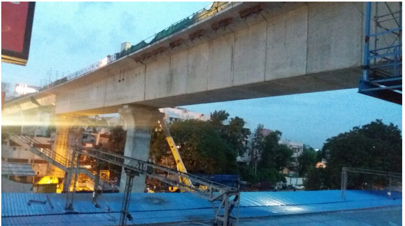
Completed view of Begumpet Metro ROB using Bridge Builder, over the Railway tracks and Railway station
