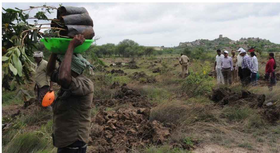
MD, HMRL Mr. NVS Reddy inspecting the preparatory works at Centre for High Energy Systems & Sciences (CHES) in Kanchanbagh
