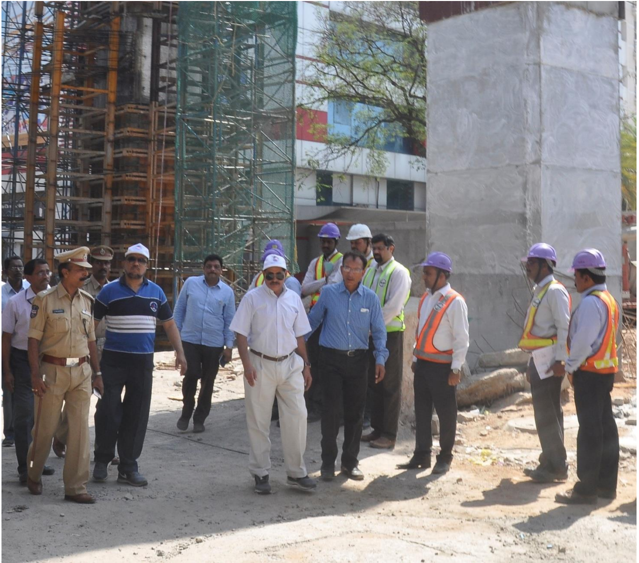
MD, HMRL Mr. NVS Reddy inspecting the Rail Over Bridge (ROB) works at Begumpet on Monday (April 25, 2016)
