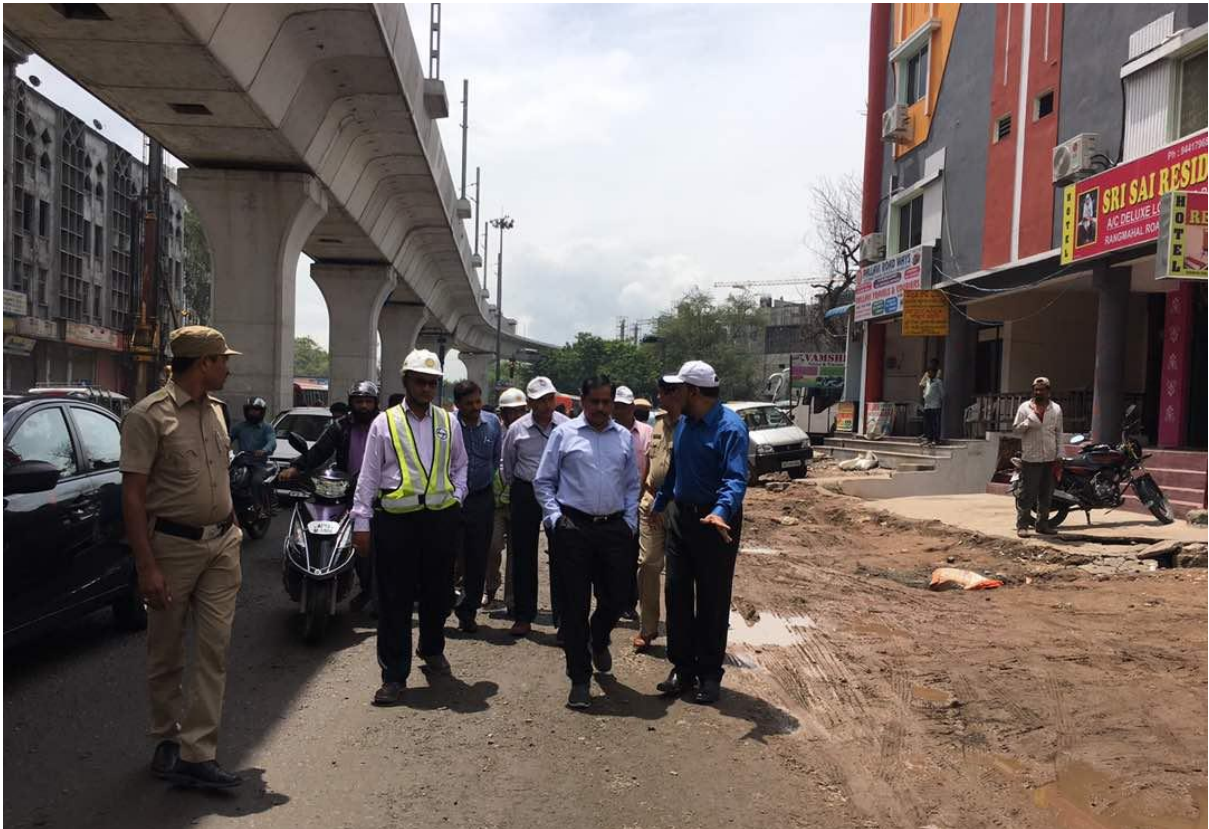
MD, HMRL Mr. NVS Reddy inspecting monsoon related works at Rangmahal junction near Putlibowli/MGBS today (Tuesday).
