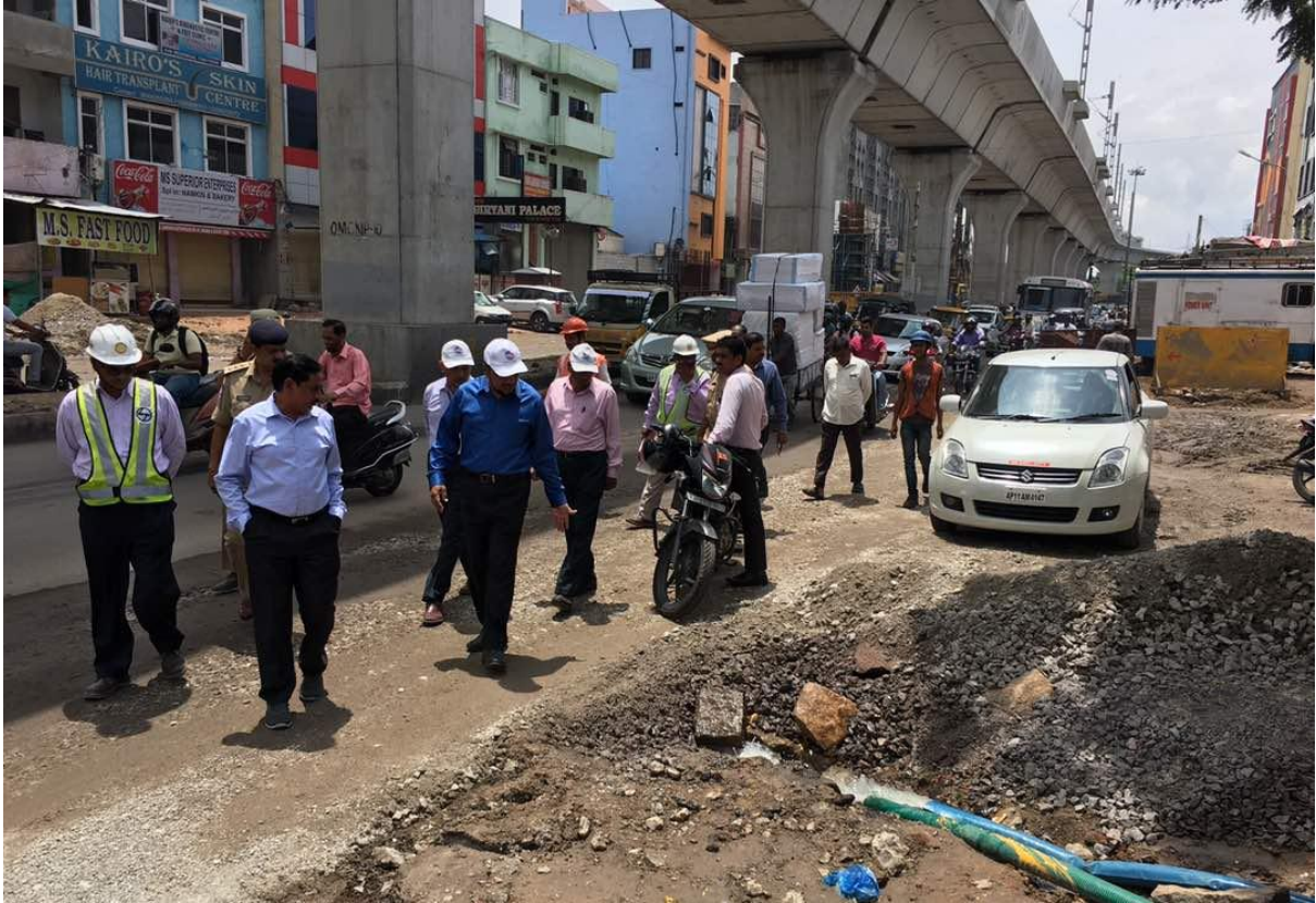
MD, HMRL Mr. NVS Reddy inspecting monsoon related works near Metro Rail station near Osmania Medical College today (Tuesday).
