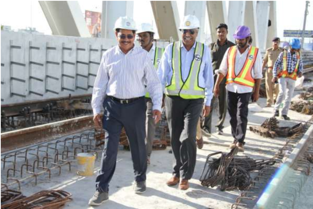
MD, HMRL Mr NVS Reddy along with MD, L&TMRHL Mr Shivanand Nimbargi inspecting the track and deck works atop Oliphant Metro ROB on Sunday (10.09.2017)
