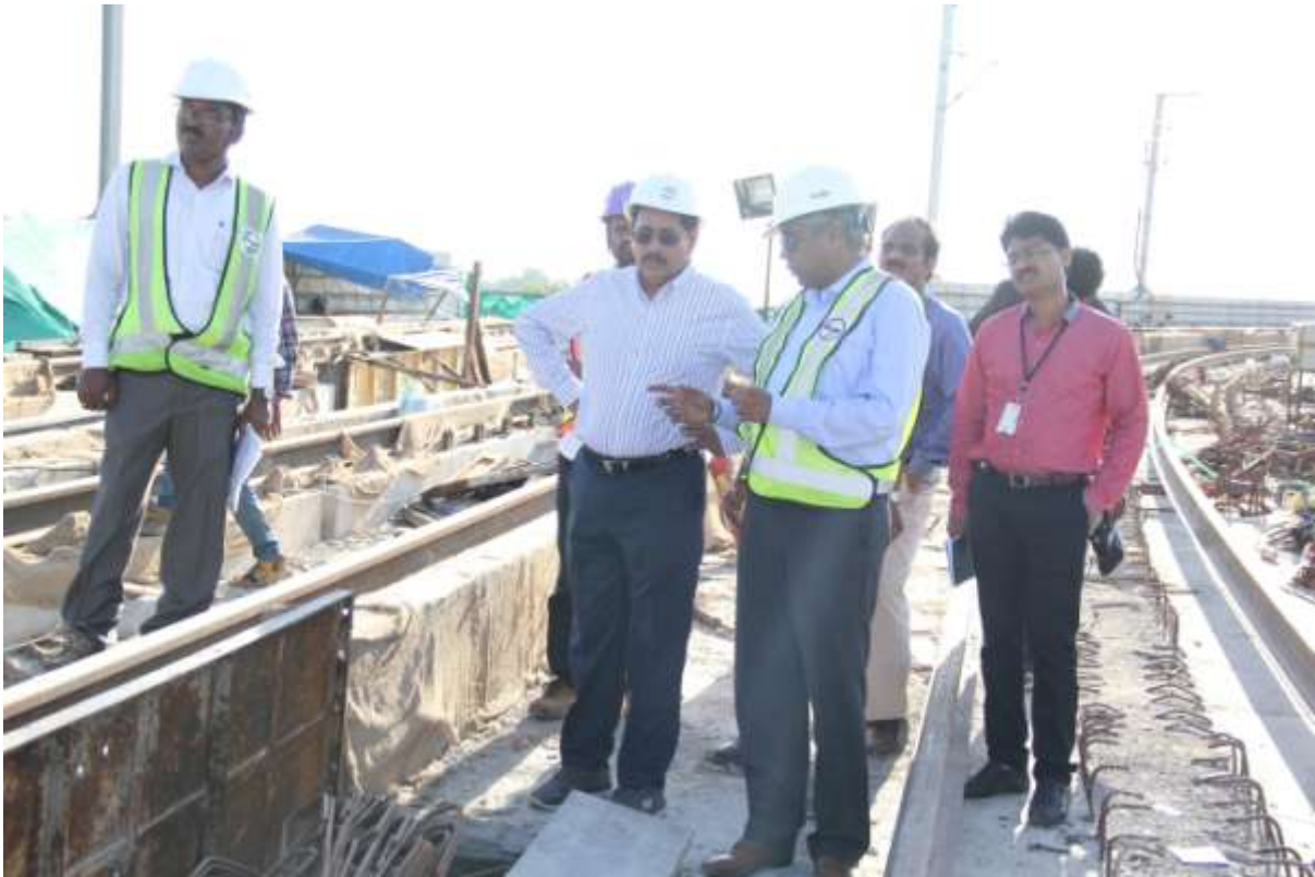
MD, HMRL Mr NVS Reddy along with MD, L&TMRHL Mr Shivanand Nimbargi inspecting the track and deck slab works atop Metro viaduct on Sunday (10.09.2017)
