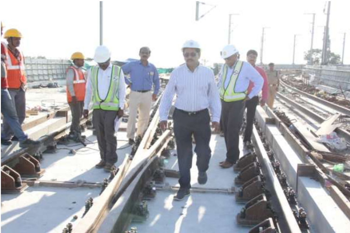
MD, HMRL Mr NVS Reddy inspecting the track works atop the Metro viaduct on critical stretches on Sunday (10.09.2017)
