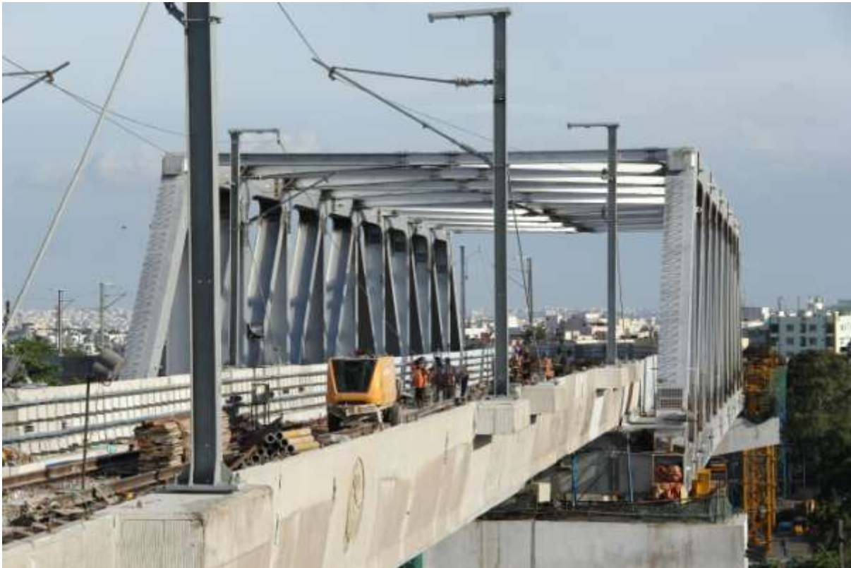
Magnificent view of recently constructed Oliphant Metro ROB on Metro corridor III (Nagole-Hitec city)
