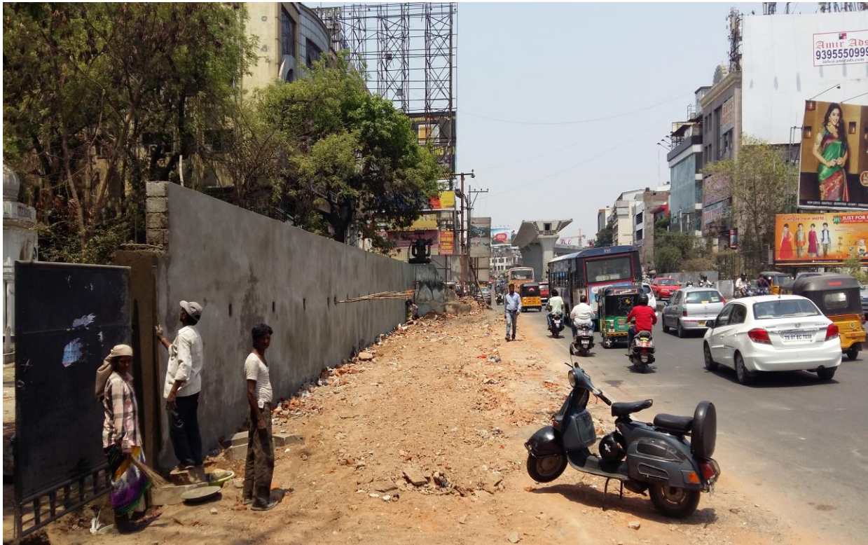
Demolition of old compound wall of a graveyard and widening of road (by 16 ft) in between two graveyards in the narrow Srinagar Colony junction, Punjagutta
