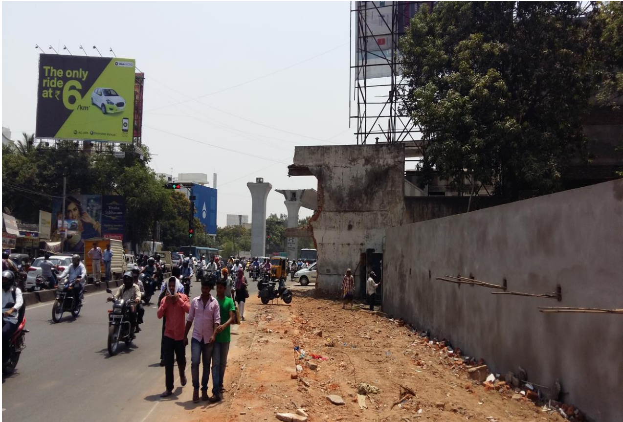
Demolition of old compound wall of a graveyard and widening of road (by 16 ft) in between two graveyards in the narrow Srinagar Colony junction, Punjagutta
