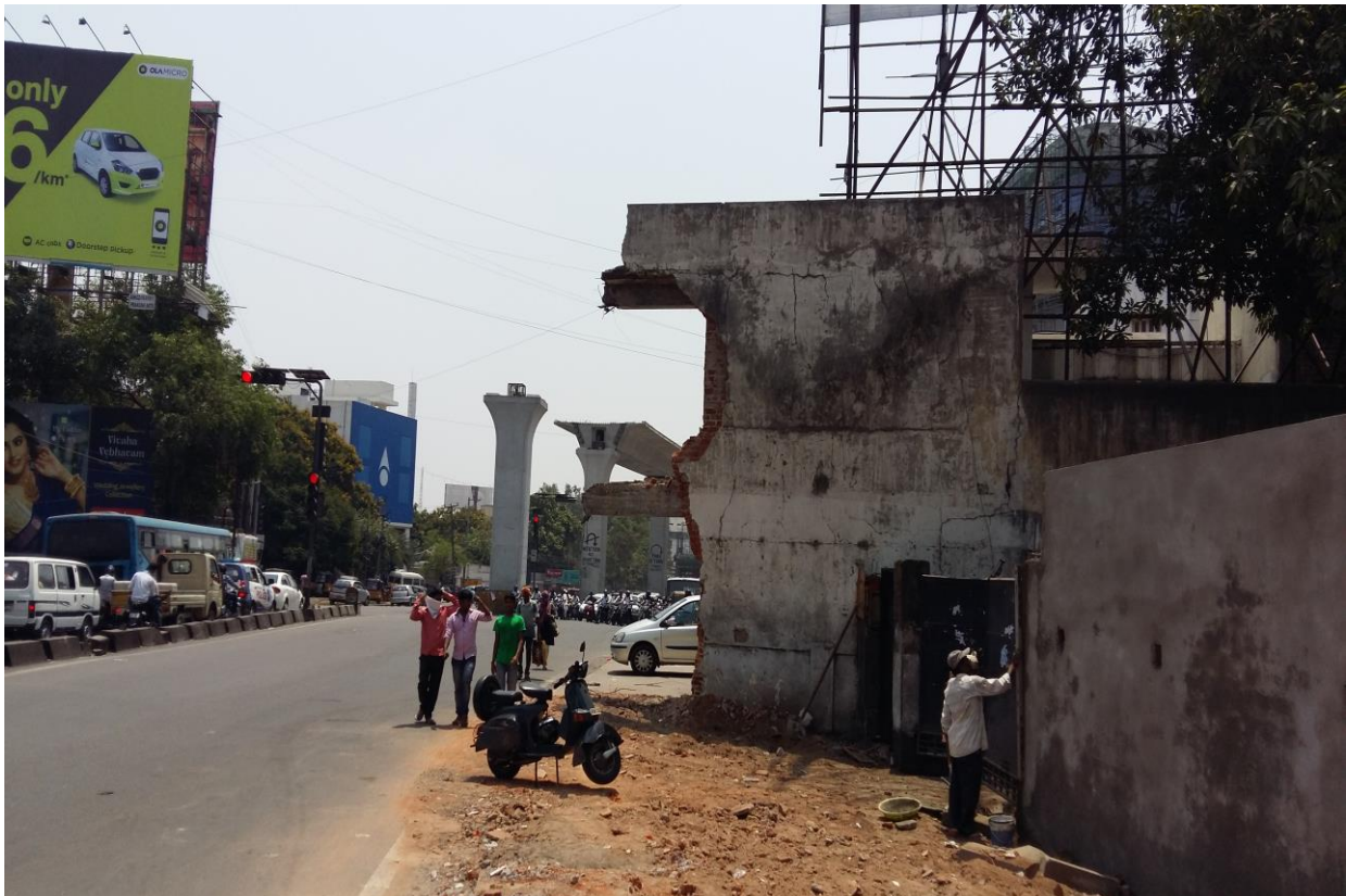
Demolition of old compound wall of a graveyard and widening of road (by 16 ft) in between two graveyards in the narrow Srinagar Colony junction, Punjagutta
