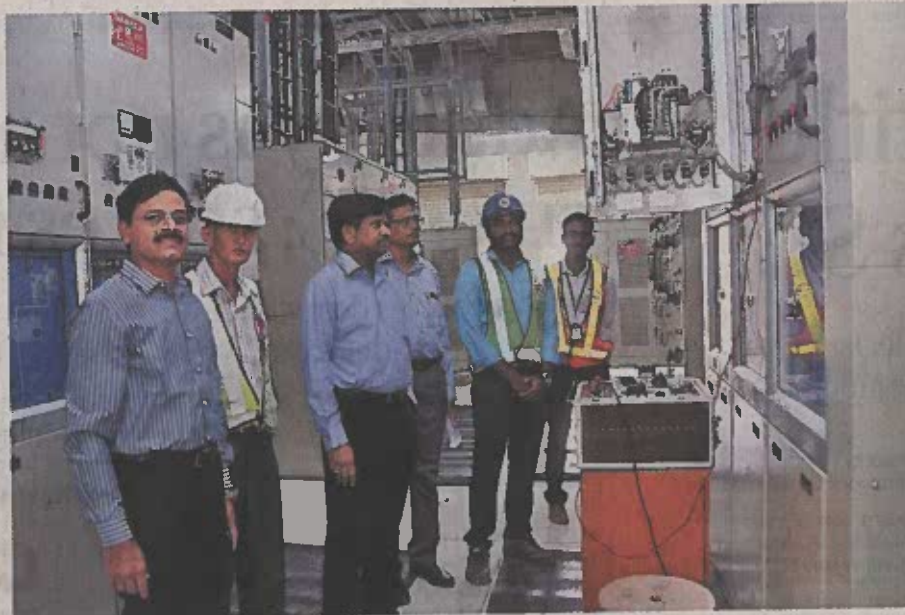
D.V.S. Raju, Chief Electrical Inspector to Government of India for HMR project, along with other officials inspecting an auxiliary substation in the city on Thursday. • BY ARRANGEMENT
