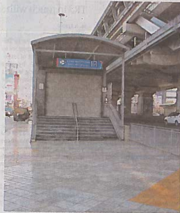
Street-level work in progress under a metro station in the city on Sunday. • BY ARRANGEMENT
