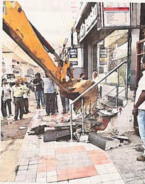
Staircase of a commercial establishment being demolished on the Malakpet-LB Nagar stretch of Metro Rail corridor.
