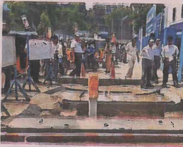
WATER CONSERVATION: Each rainwater harvesting pit with injection borewell costs Rs 1.5 lakh.
