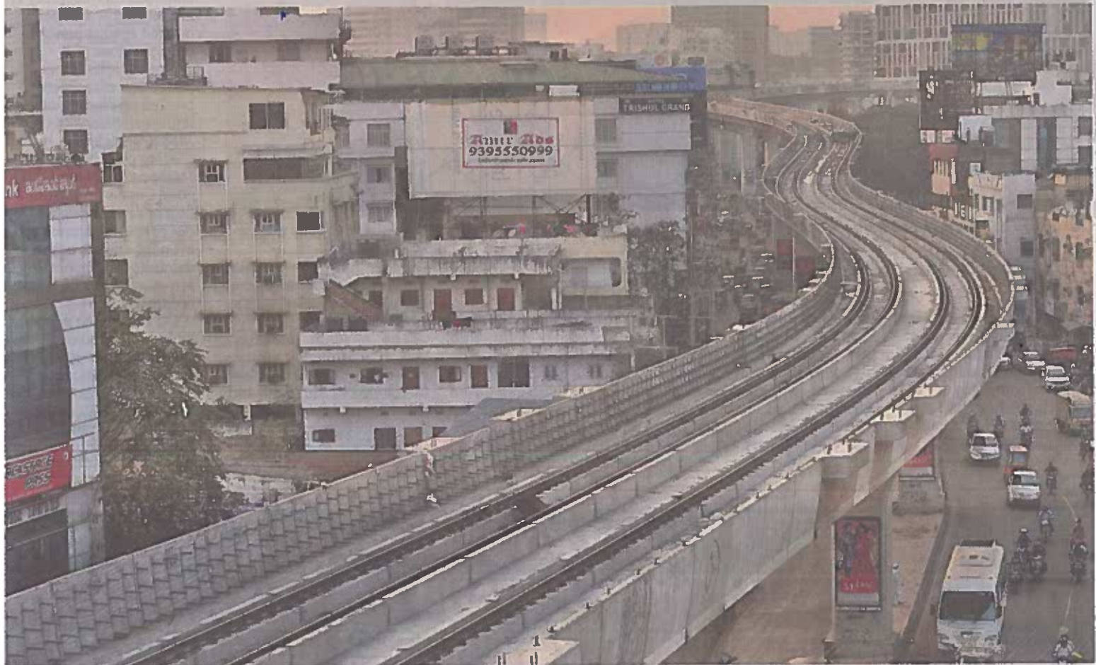
Metro Rail works are under progress on the Jubilee Hills Checkpost-Cyber Towers route. — Photo: Hrudayanand
