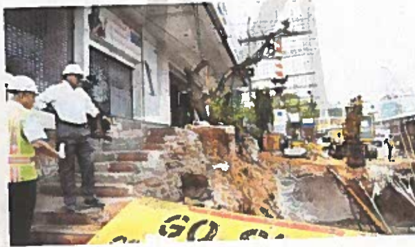
MOVING FORWARD: Preparation for the Hyderabad Metro Rail project viaduct at Begumpet in Hyderabad. — PHOTO: BY ARRANGEMENT
