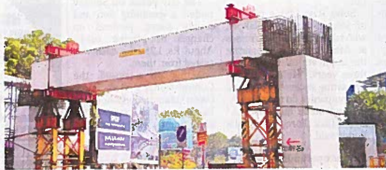
L&T Metro Rail adopting pre-cast type of construction for flow of traffic down below. - PHOTO: MOHAMMED YOUSUF
