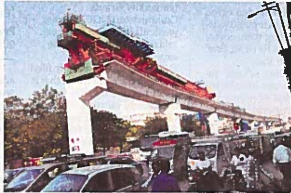
Construction work of Metro Rail on corridor-III has been put on fast track. - PHOTO: MOHAMMED YOUSUF
