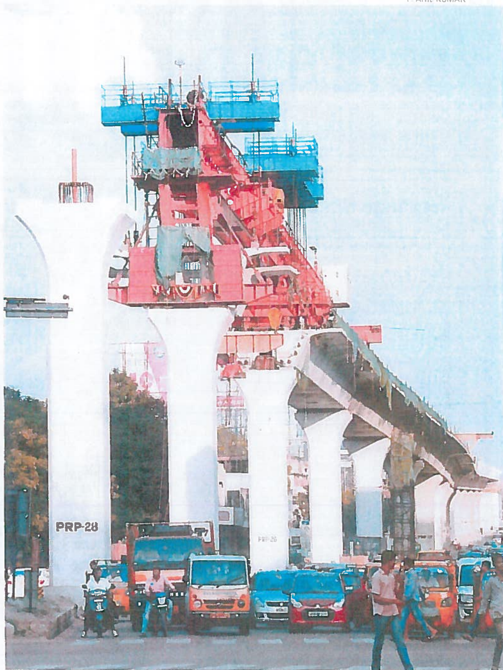
Sleeper cell A stalled section of the Metro work in Hyderabad
